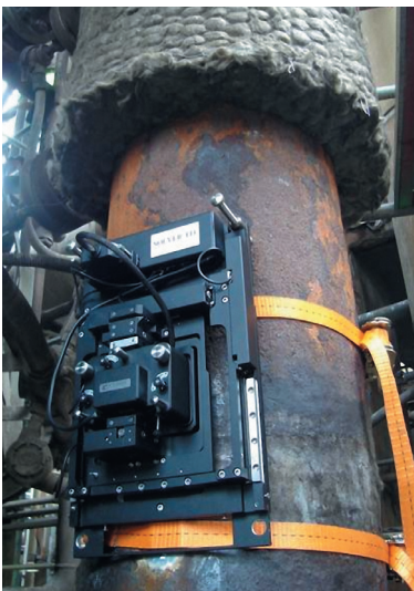
SPM mounted on a pipe
